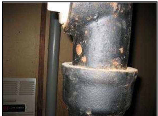
3.0 Picture 4 Main Stack Seepage Barnacles
