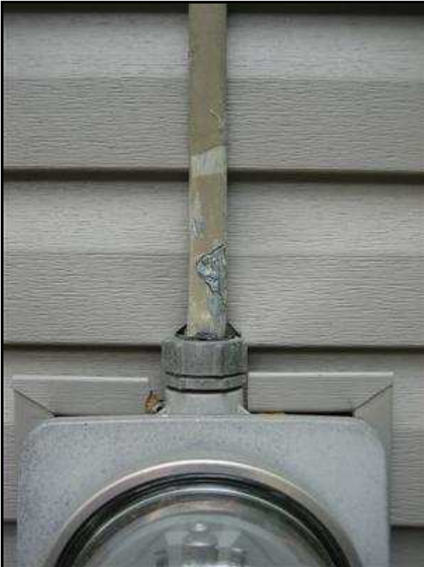
3.0 Picture 1 Damaged SE Cable
