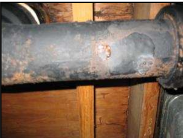
3.0 Picture 3 Main Stack Closet Bend
