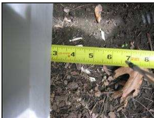
3.0 Picture 7 Tape measures 2 3/4 inch to foundation wall at left center of rear wall bottom of siding.
