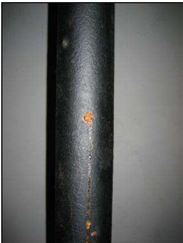
3.0 Picture 5 Main Stack Seepage Barnacles
