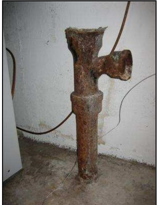
3.0 Picture 2 Corroded Standpipe
