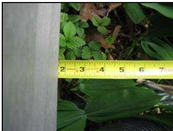
3.0 Picture 6 Tape measures 1 3/4 inch to foundation wall at bottom of siding near SW corner rear wall.
