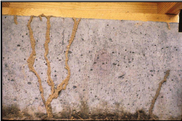
Termite Shelter Tubes
